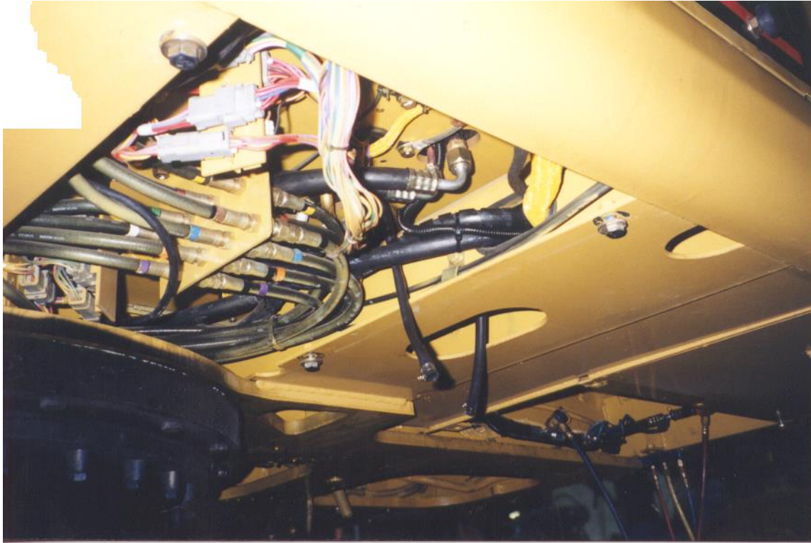
View showing underside of evaporator area with hose assemblies and drain tubes.
